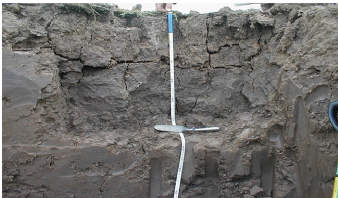
Fig. 1. Exposed fissures through trenching on the disused Thorngumbald embankment (after Dyer et al., 2009).
