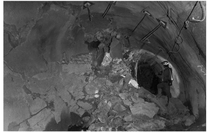
Fig. 2. Localized damage to a mine tunnel (Ortlepp, 2000).
