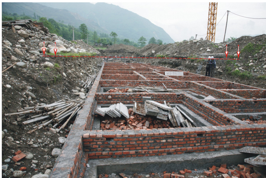
Fig. 2. A row of houses built within a surface rupture zone without considering a safety distance: arrows showing the rupture scarps.
