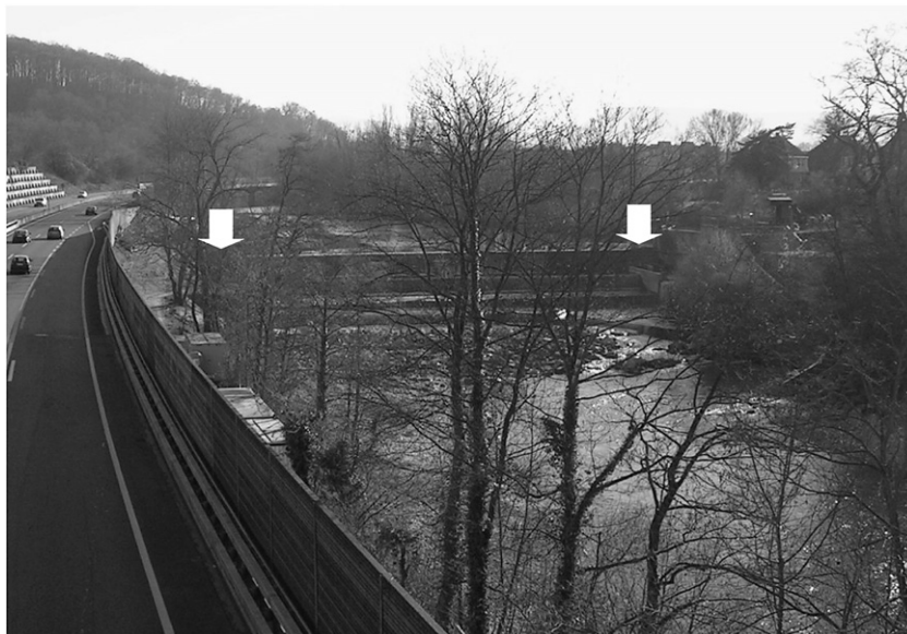
Fig. 1. An overview photo of the dam structure on the Birs river, Neuwelt, Basel, Switzerland. The gray arrows mark the east and the west bank of the river (left to right on the photo). The camera is directed towards south–south west.
