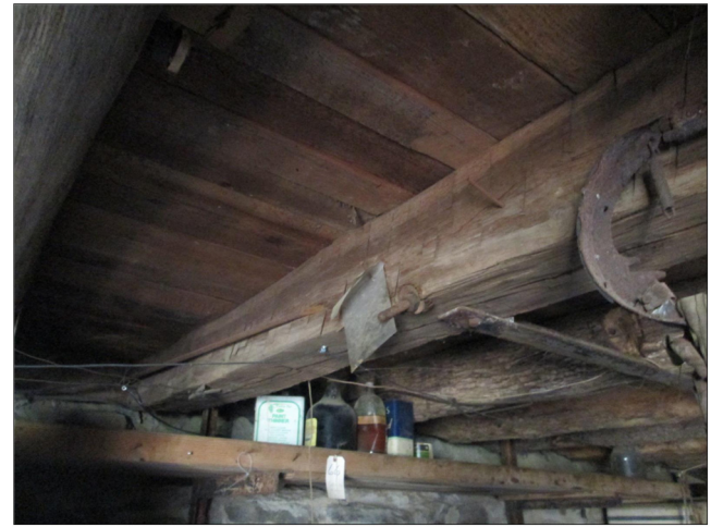
Fig. 2. First floor joists accessible in the cellar. The log in the center is hand-hewn while the log behind and to the right is un-hewn with intact bark.
