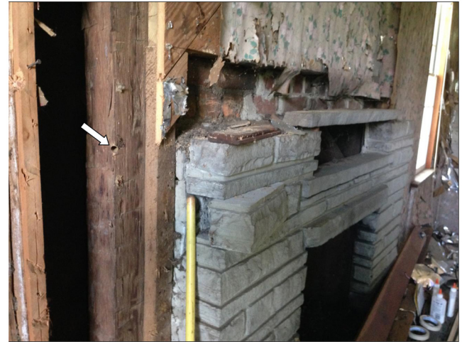
Fig. 3. Location of sample SH1005 (arrow) showing how most of the beams we sampled on the first and second floors of Sabine Hill had been squared during fabrication.
