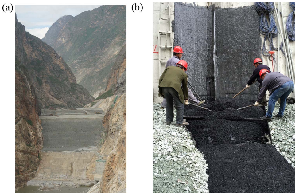
Fig. 1. (a) The 174-m high Quxue Dam under construction; (b) asphalt core-plinth connection on the dam left abutment with a slope of 1 V: 0.33H ( 72^\circ ).
