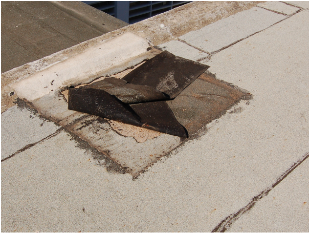
Fig. 1. Example of a failed waterproofing membrane repair.
