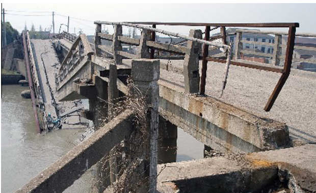
Fig. 1. Sudden collapse of Yanyue Bridge in Wujiang, China [21,22].
