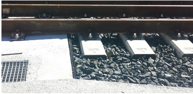
Fig. 1. Track separation in slab track (left) and ballast track (right) in a track transition.
