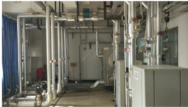
Fig. 1. Photo of the ground source heat pump located at Wuhan University of Science and Technology.
