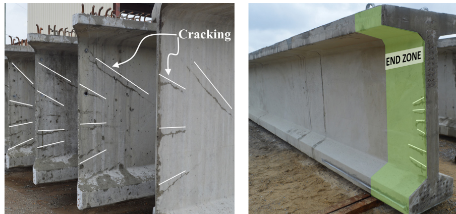
Fig. 1. Cracking observed in end zone region of bulb-tee (BT) girders stored at a precast yard.
