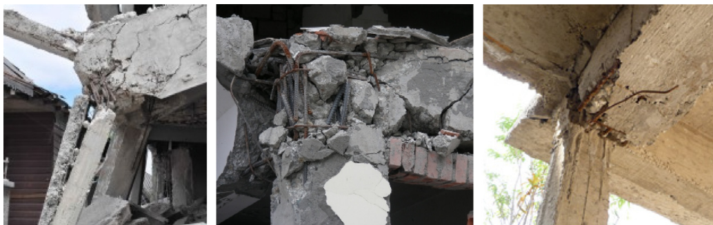
(a) Insufficient anchorage length (b) Unconfined connection (c) Poor coverage
