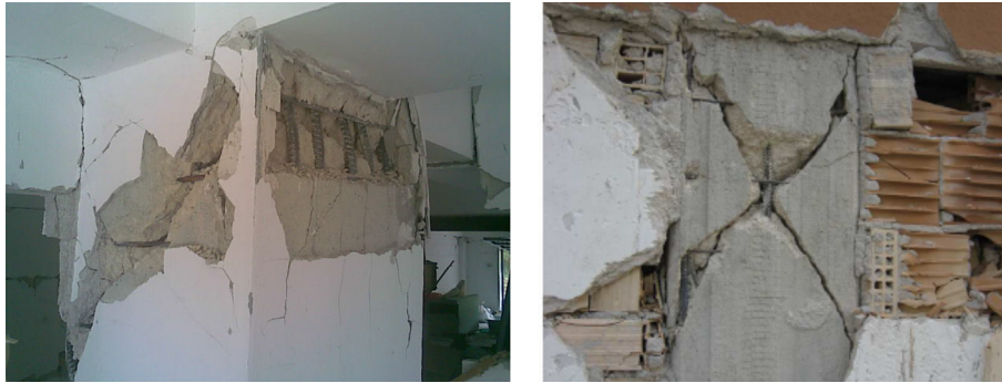
Fig. 1. Column shear failures after L'Aquila earthquake, 2009, Italy.
