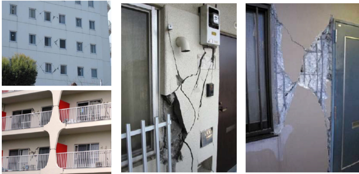
Fig. 1. Damage of lightly RC walls after the 2011 Tohoku Earthquake.
