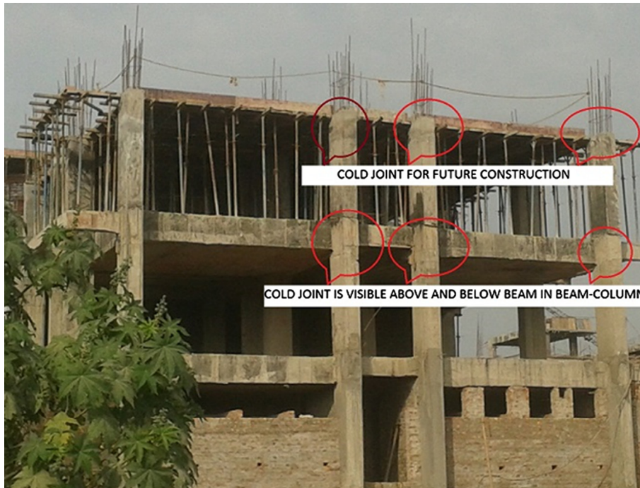
Fig. 1. Photograph of in-situ construction with cold joint in column.
