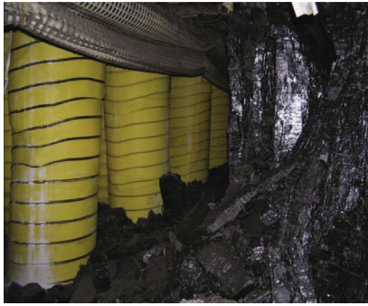
Fig. 1. Pumpable roof supports in a longwall recovery room.
