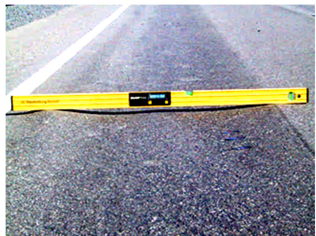
Fig. 1. A view of the rutting occurrence in asphalt pavement.
