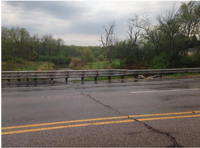
Fig. 1. Typical thermal cracking in asphalt pavements.
