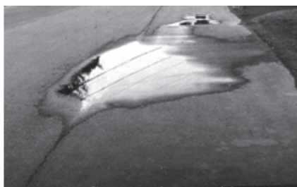
(a) Slippage Failure
