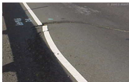
(b) Surface Layer Delamination
