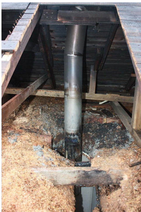
Fig. 1. Chimney roof penetration after fire.
