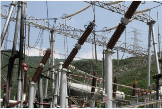
Fig. 2. Failure of 220 kV porcelain surge arresters in 2008 Wenchuan Earthquake [8].
