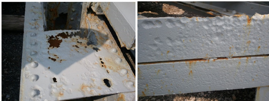
(b) Pictures of the corroded members of the Yeongdo Bridge
