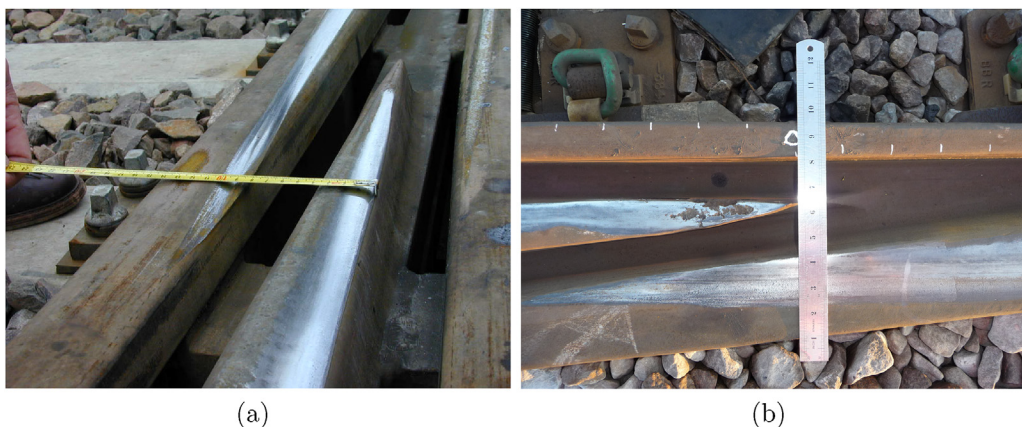
Fig. 2. Examples of damage in a railway crossing: (a) plastic deformation of the wing rail and (b) rolling contact fatigue of the crossing nose (spalling). Photos published with permission from (a) voestalpine VAE GmbH and (b) Jay Jaiswal, private communication.
