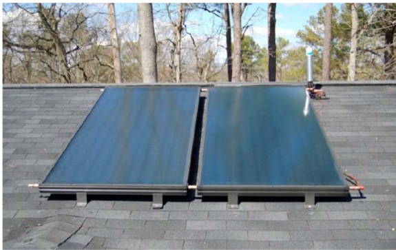
Fig. 1. Roof-mounted, flat-plate solar collector.
