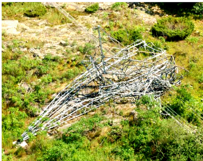
Fig. 1. Guyed tower failure in Ontario, (Hydro One Report, 2006).
