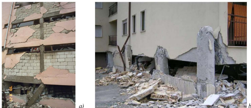
Fig. 2. Local failures of RC frames due to the interaction with infills: a) Failure of a joint; b) Failure of a column end; c) Failure of column and joint.
