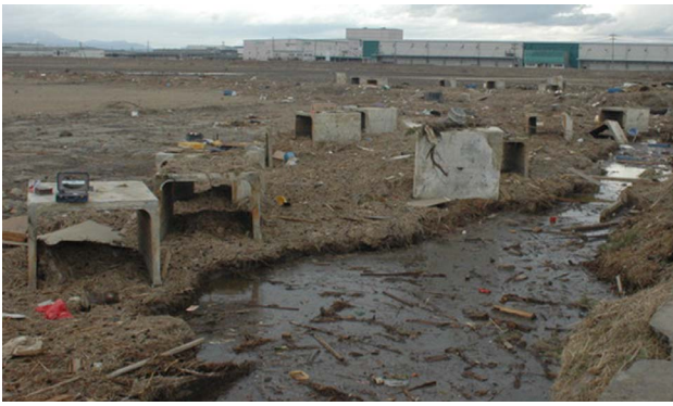
Fig. 1. Ground damage and floatation of U-shaped water tubes due to liquefaction in the 2011 Great East Japan Earthquake (Chian and Tokimatsu, 2012).
