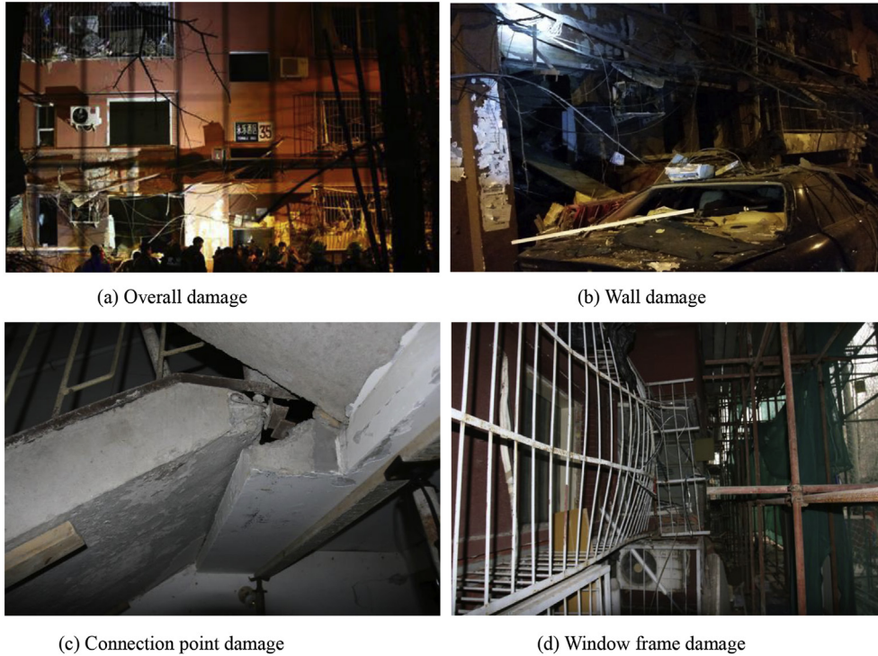
Fig. 1. Damage to building structures.
