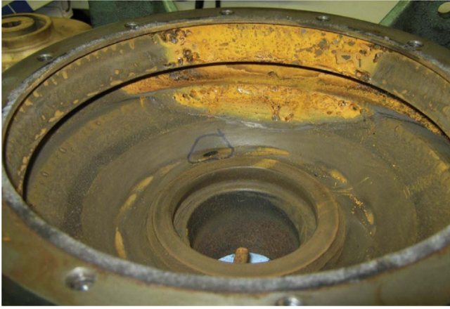
Fig. 1. Erosion wear on centrifugal pump casing at actual site.
