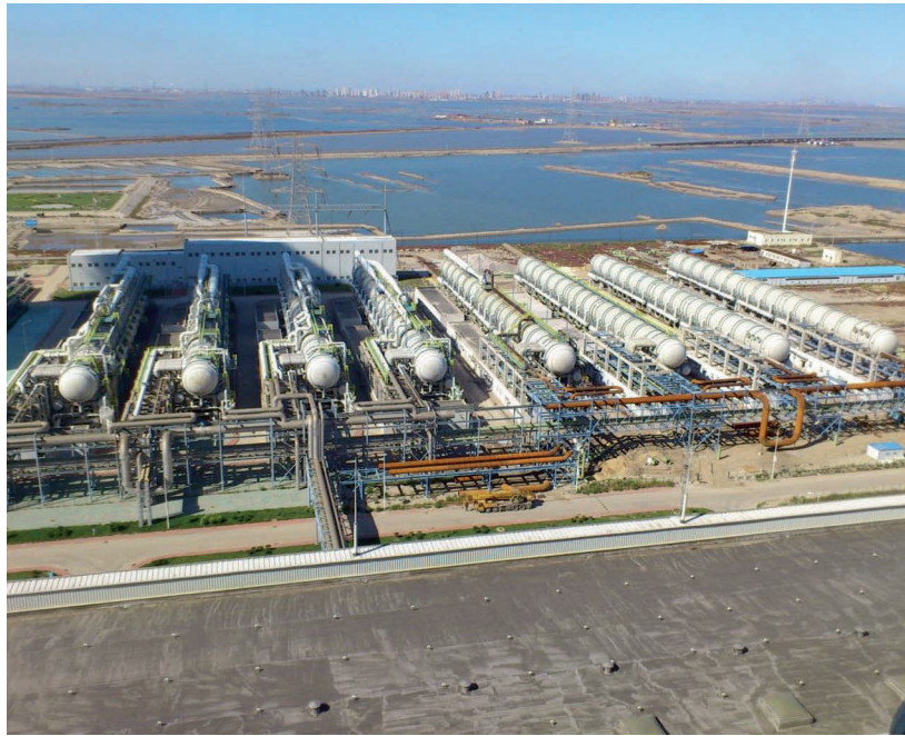
The Tianjin co-located plant in China (Image: IDA)
