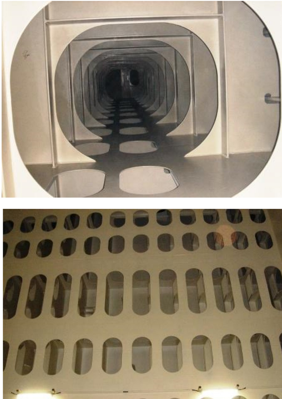
Fig. 1. Examples for free edges in maritime steel constructions.
