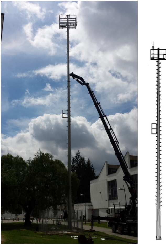
Fig. 1. Installation of the 30 m high Corona current measuring mast in the campus of the Universidad Nacional de Colombia.
