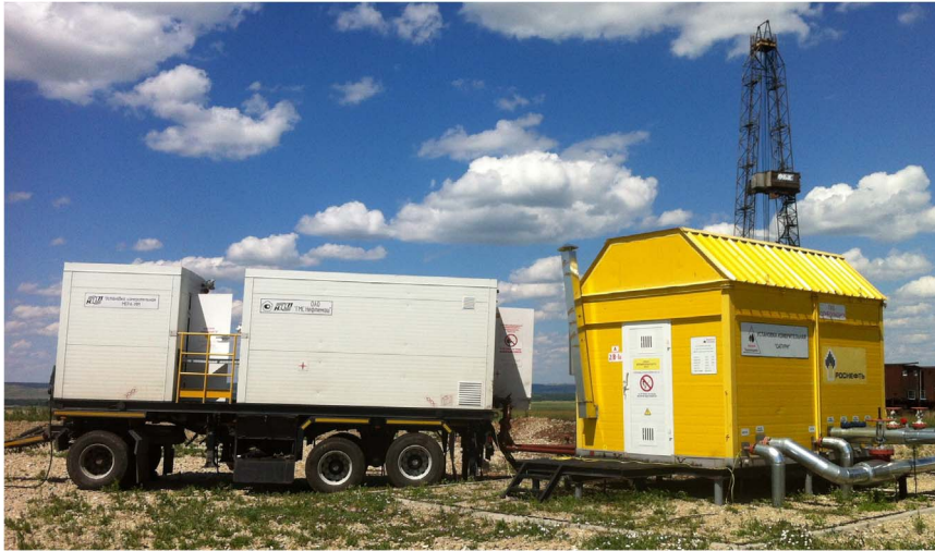
Fig. 1. (Right) conventional well test station, including separator. Note piping to handle multiple well production streams. (left) Mobile trailer carrying NOG system. Note piping extended from well test station, enabling NOG system to perform well tests.
