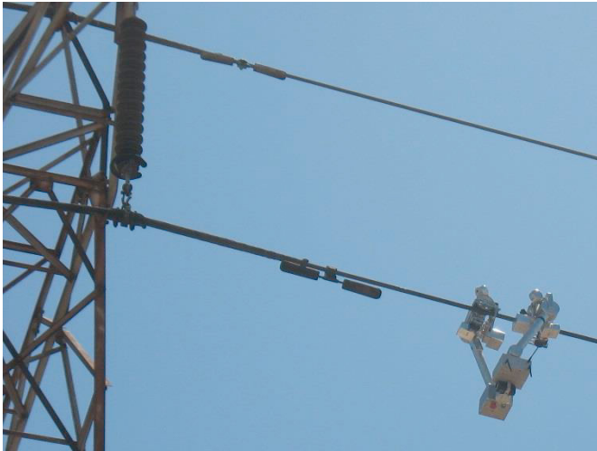
Fig. 2. Power line robot deployed on a single-conductor 132 kV line showing the normal rolling configuration
