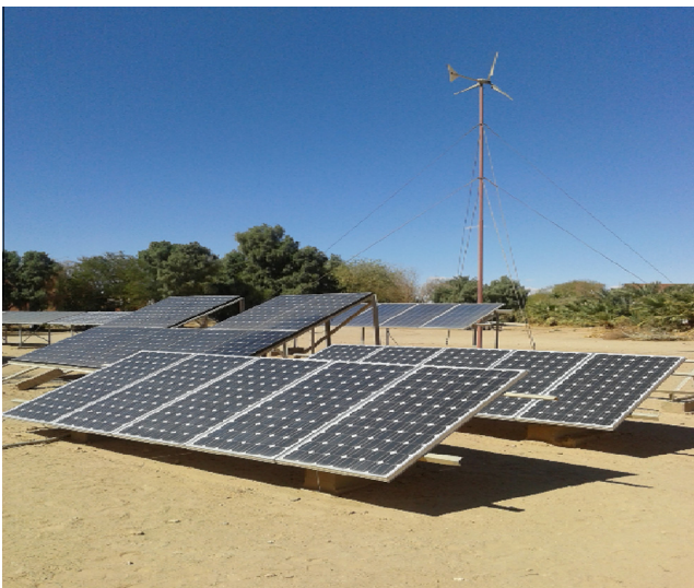
Fig. 1. View of the 1.75 kW PV plant installed in field of URERMS, Adrar.
