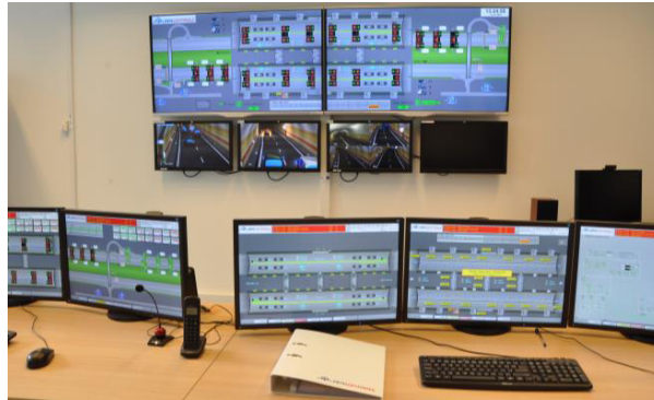
Fig. 1. Tunnel Traffic & Operation Simulator.
