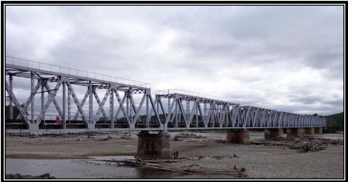
Fig. 1. General view of the bridge across the Amgun’ River. The riverbed part of the bridge crossing is set up of quaternary alluvial deposits. Steel trusses with parallel chords; deep foundations and supports are built of site concrete.
