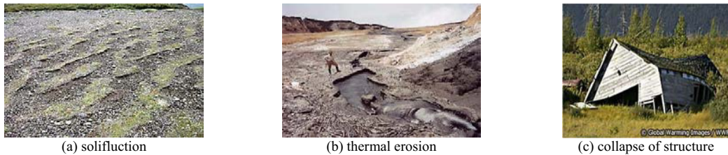
Fig. 1. Damage caused by the thawing of permafrost
