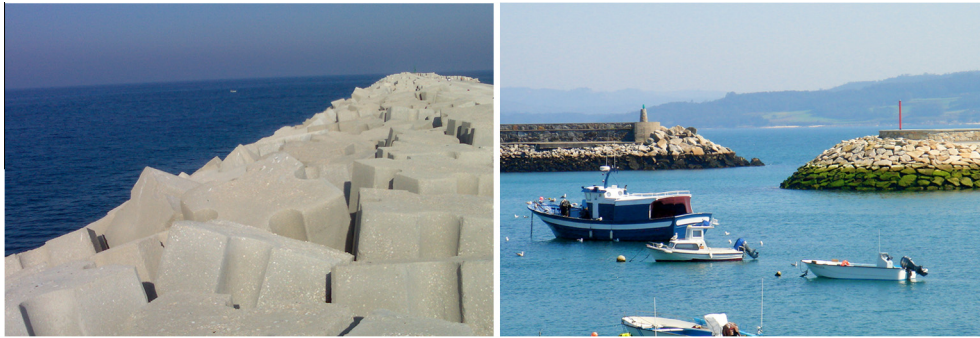
Fig. 1. Pictures of the antifers breakwater in Molfetta (Italy) and rubble mound breakwater in Muxía (Spain).
