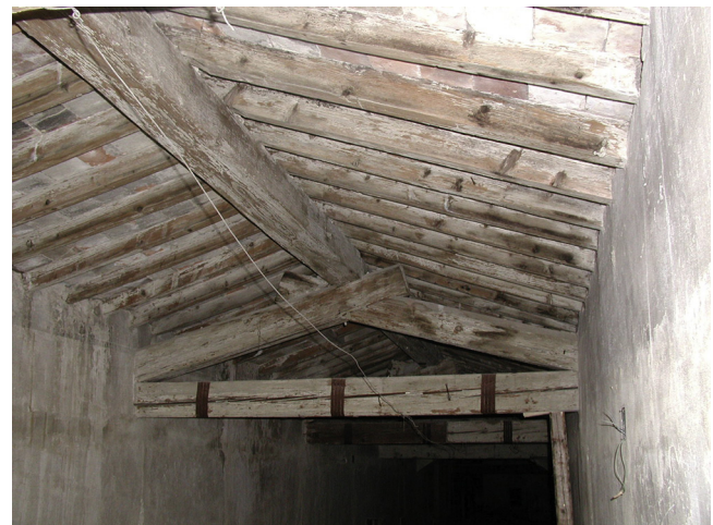
Fig. 1. Absolutely useless fastening with iron strap of a truss tie affected with a check caused by shrinkage (Villa Demidoff, Florence. Photo Tampone).
