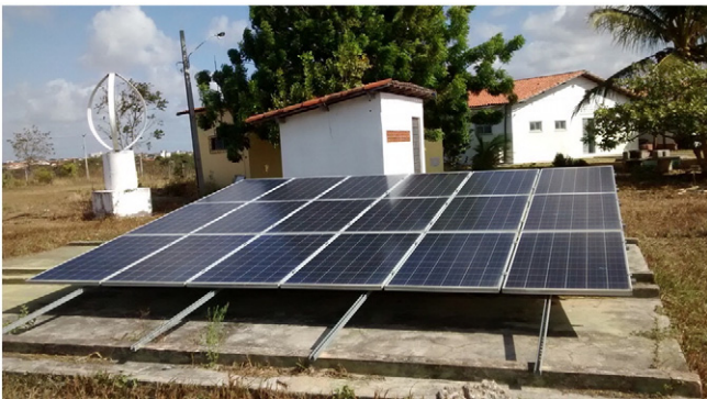
Fig. 1. Picture of the PV array used.
