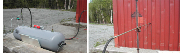
Fig. 4 – Gas storage tank and fuel supply system.
