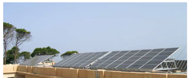
Fig. 1. The PV array installed on the roof of the CDER building in Algiers, Algeria (Arab et al., 2005).
