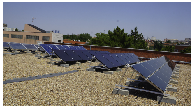
Fig. 1. Experimental portion of the grid-connected roof-standing solar plant in ETSIAAB (Madrid, Spain).
