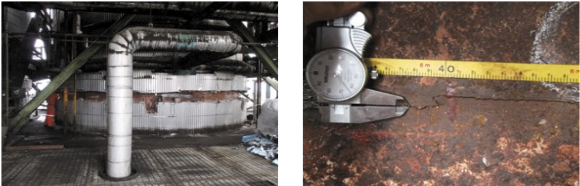
Fig. 1. Left: Coker drum with the thermal insulation removed in the skirt junction. Right: Cracking of the skirt junction running along the weld line in the skirt side.
