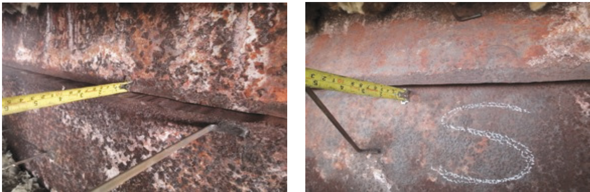
Fig. 2. Misalignment of the fractured edges of the skirt junction.
