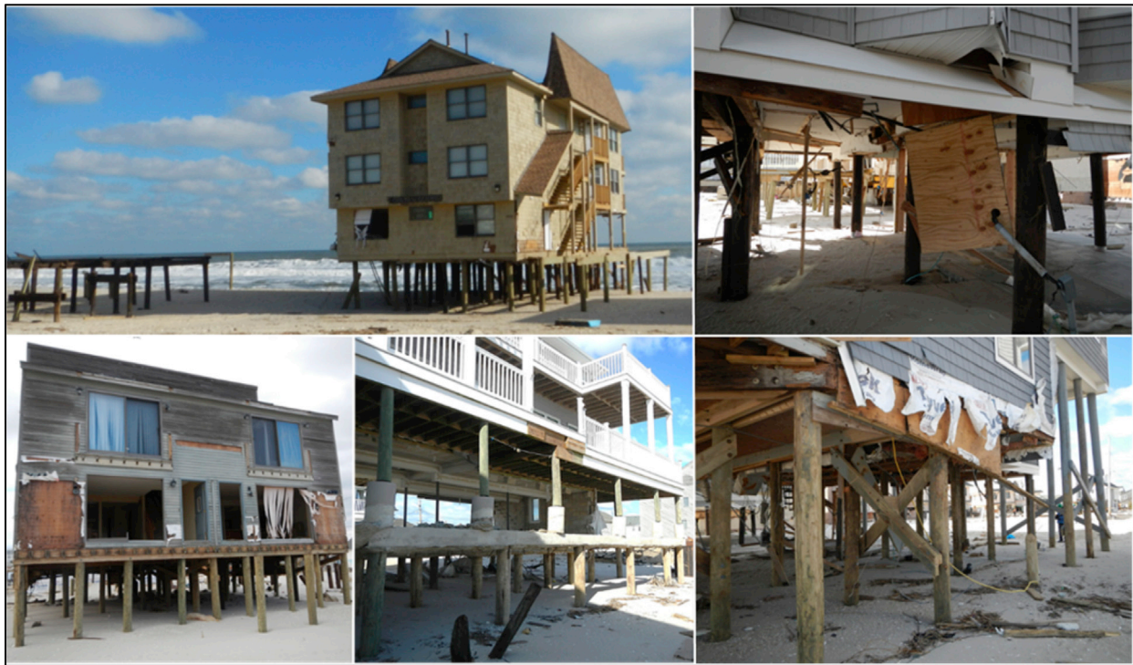
Fig. 1. Examples of wave and surge-induced damage to elevated coastal structures located in Toms River, New Jersey occurring after Hurricane Sandy (2012). Photographs by Tori Tomiczek.
