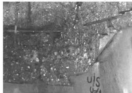
(b) Concrete exposed in eroded runner chamber
