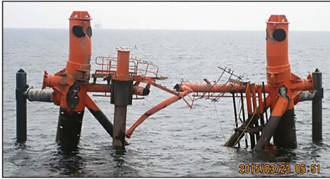
Fig. 1. South Pars SPD13-A jacket one day after accident and before collapse.
