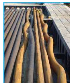
Fig.1 The picture of rod strings' buckling
