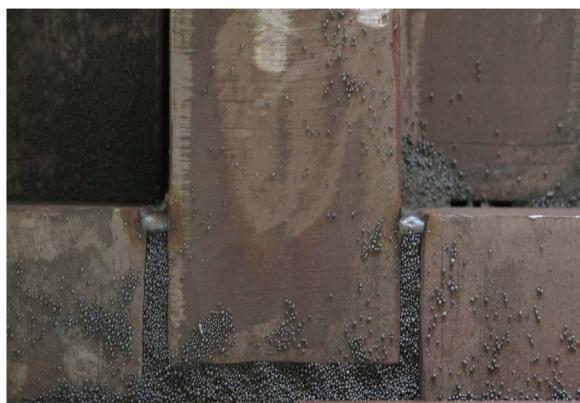
Fig. 2. Spaces in the joints of the biological shielding filled up with steel pellets.
